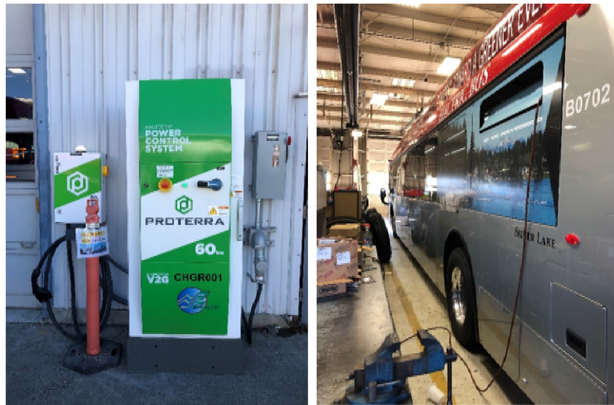
Left to right: Plug-in depot charger; Electric bus in maintenance bay with limited working space
